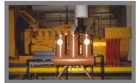
Model 3075 filtering the fuel for several stand-by generators. The product ensures ultra clean fuel when they need it. No premature filter clogging.
